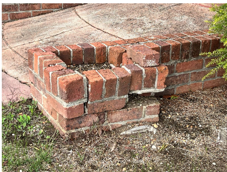
Figure 14 Damaged brick planter box.
