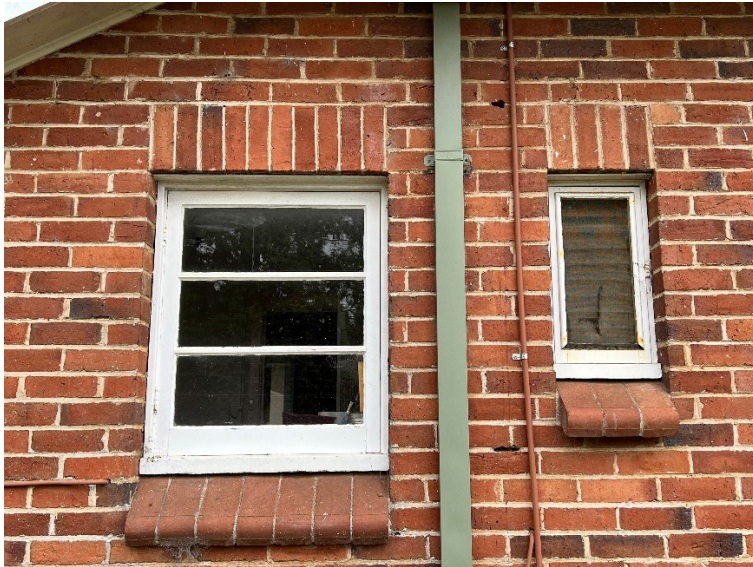
Figure 25 Multi paned timber casement window to laundry. Fixed wire mesh laminated glass louvres to WC. Mesh to flyscreen is torn.
