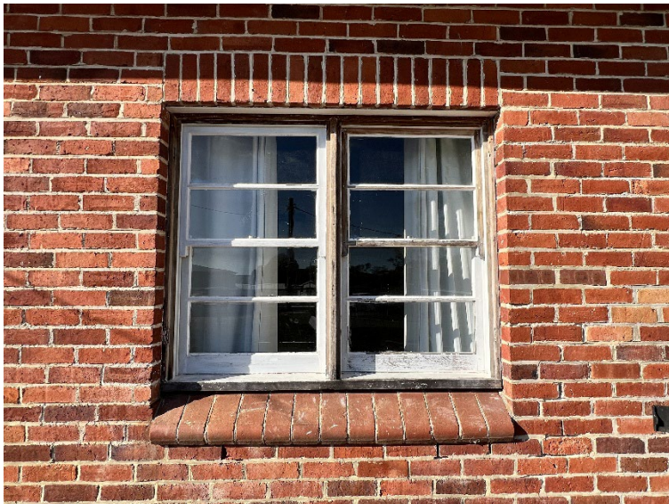
Figure 22 Two combined double hung sash windows. Timber frame and sill are showing signs of wear. Casement flyscreen missing.
