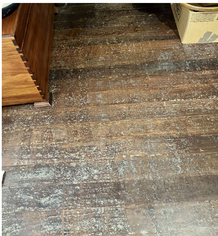
Figure 34 Carpet adhesive residue on timber floorboards.
