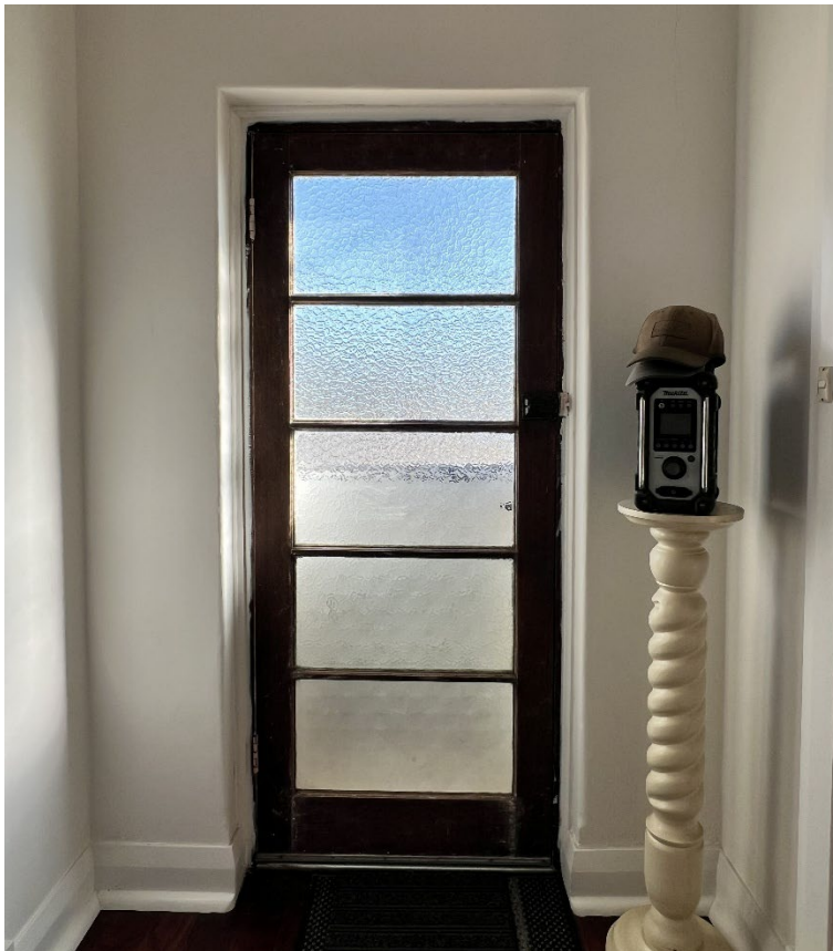
Figure 26 View of side entry door from foyer. There is a vertical crack at the top right-hand side of the wall.
