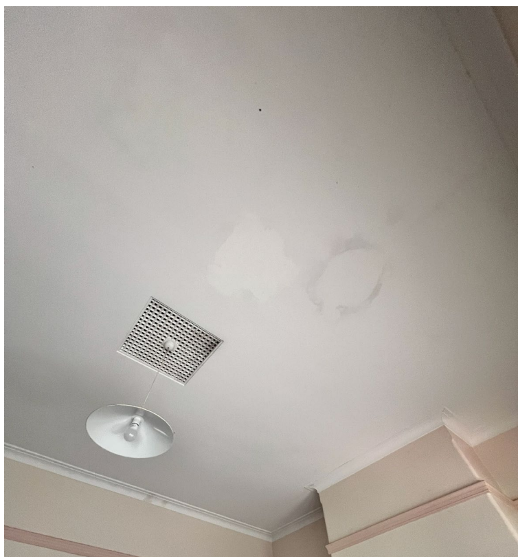
Figure 33 Small holes to ceiling. Scuff marks and stains present.
