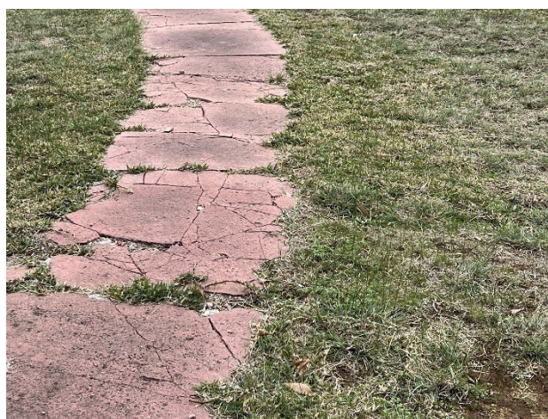
Figure 19 View showing poor condition of the concrete footpaths.
