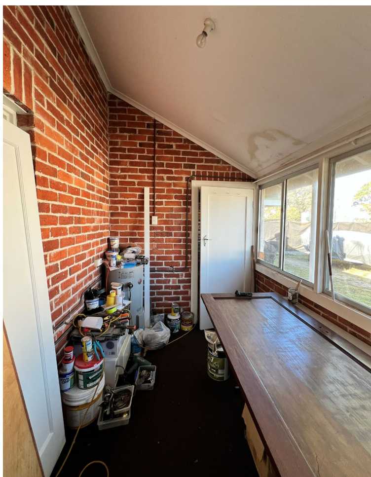
Figure 54 Water damage to ceiling.
