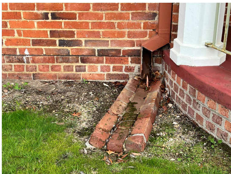
Figure 13 Damaged gutter discharging onto brick scupper drain.
