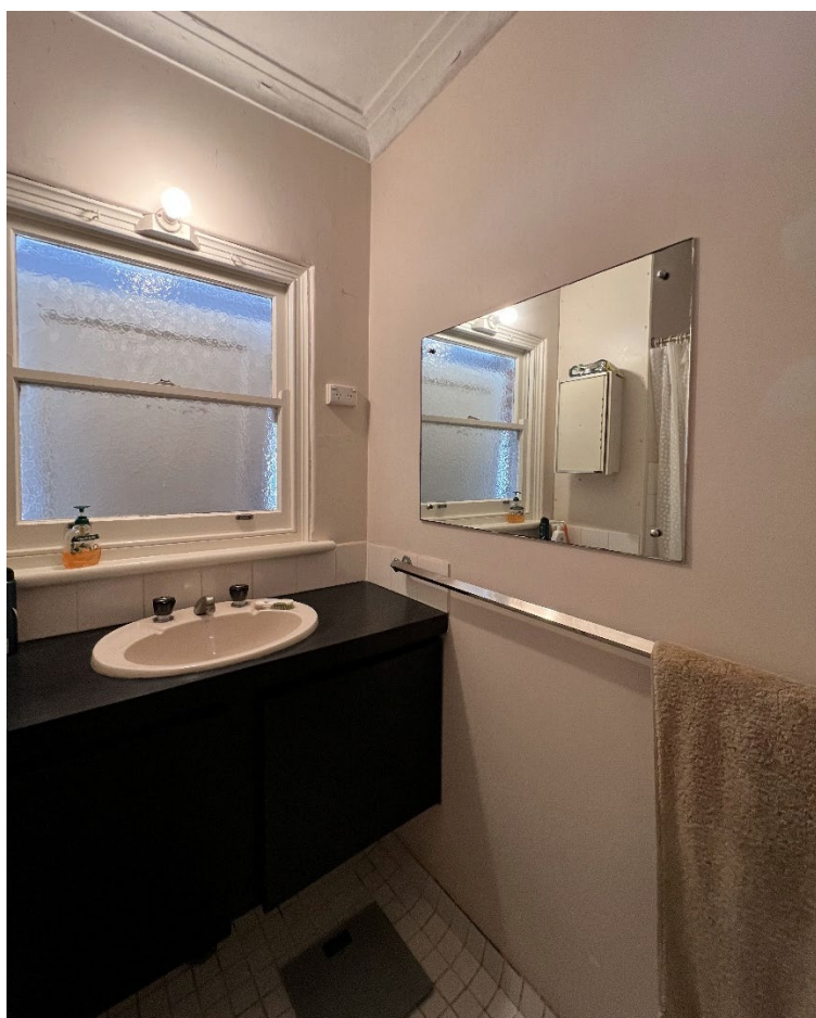
Figure 46 Paint peeling on cornices. Scuff marks on wall.
