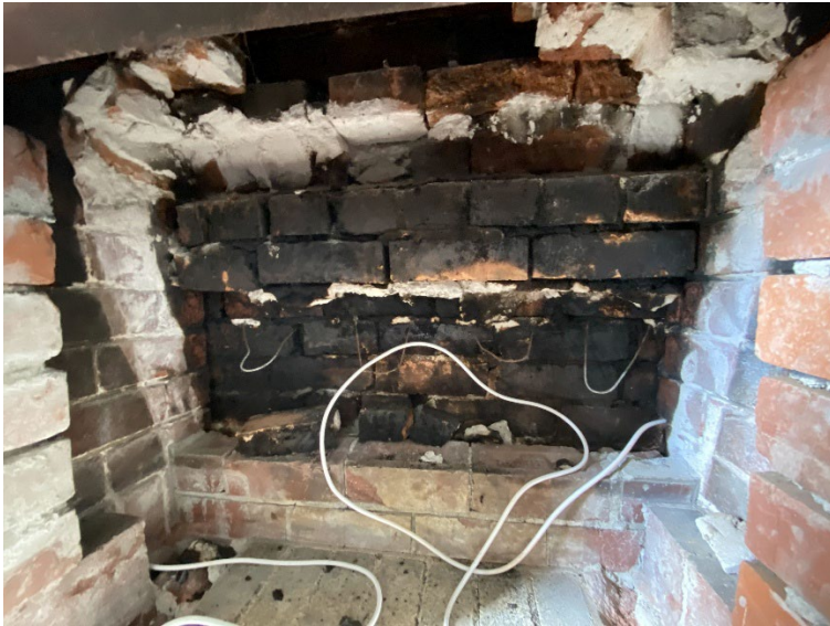
Figure 29 Internal view of firebox in living room. The firebox is severely damaged and has partially collapsed.
