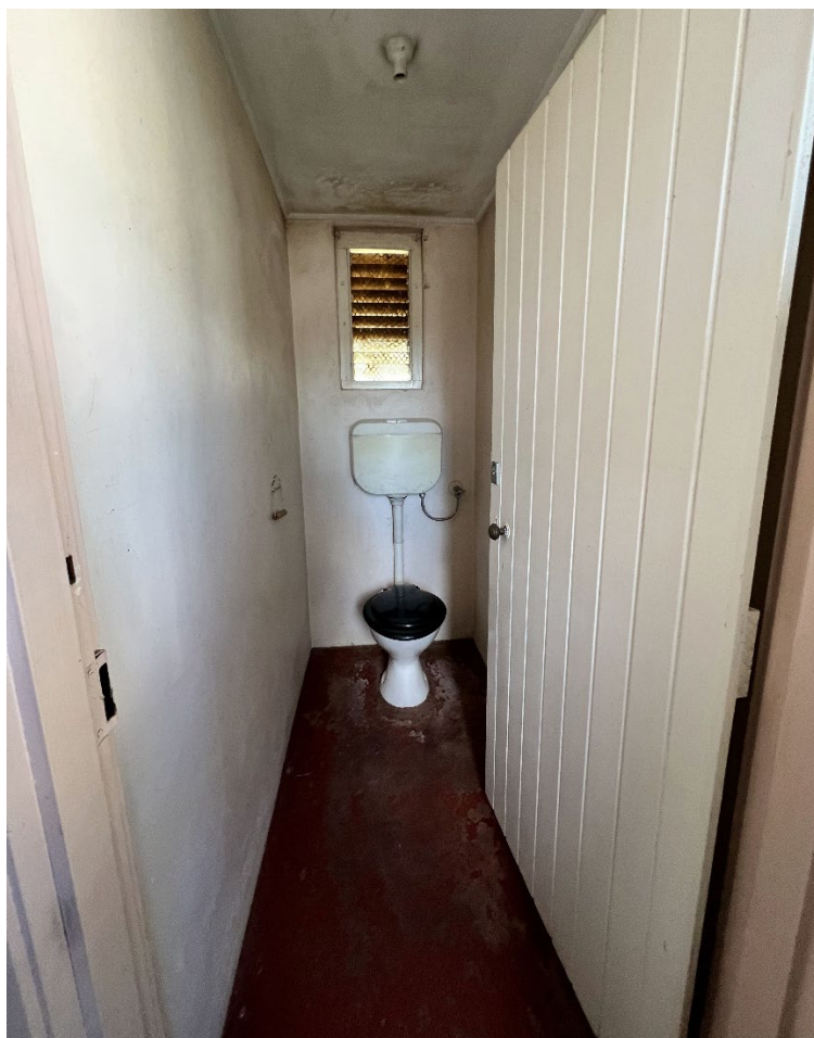
Figure 60 Plaster ceiling and walls are heavily soiled. Accumulation of dirt and grime to glass louvres. Light fitting is missing.
