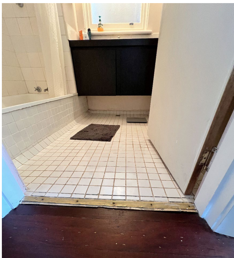
Figure 47 Transition trim is showing signs of wear. Tile grout is dirty.
