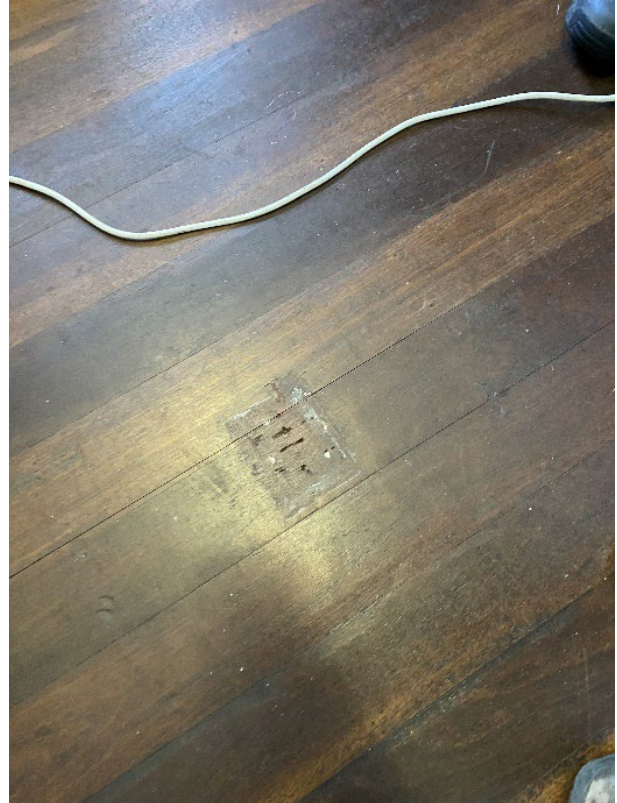
Figure 39 Evidence of central support post remaining in timber floorboards.
