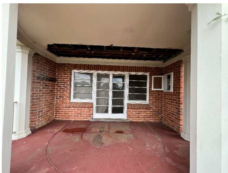
Figure 15 Collapsed ceiling to portico due to water ingress.
