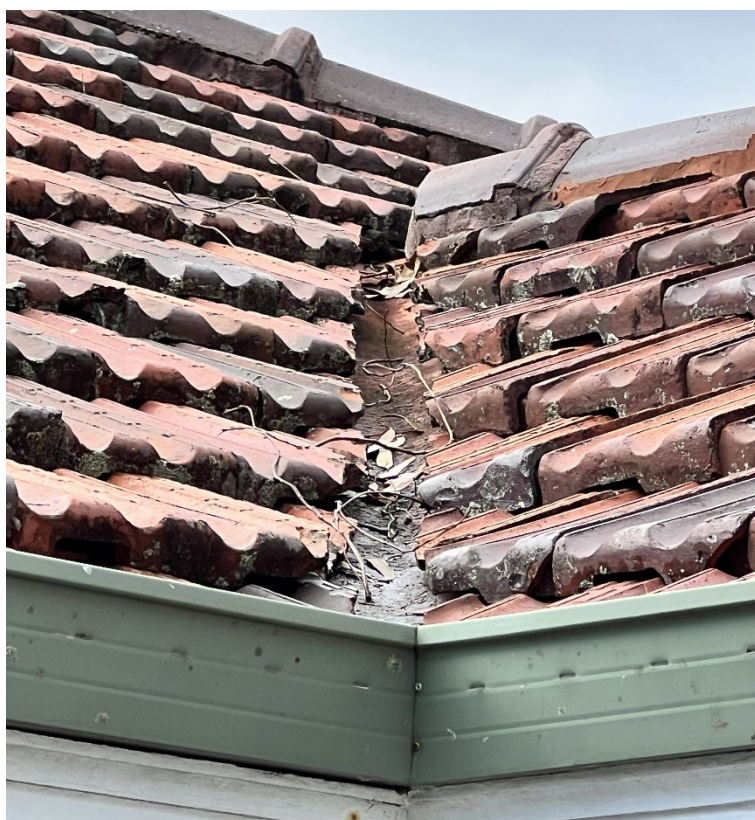
Figure 10 Valley gutter is severely deteriorated. Roof tiles have lichen growth. An accumulation of dried leaves and branches from nearby tree.
