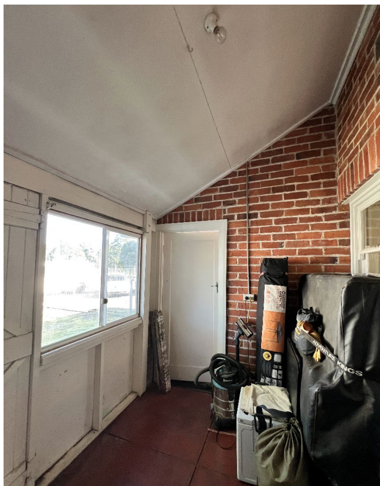
Figure 56 Asbestos sheet lining to bottom of windows. Ceiling frame visible due to accumulation of dust and grime on ceiling.
