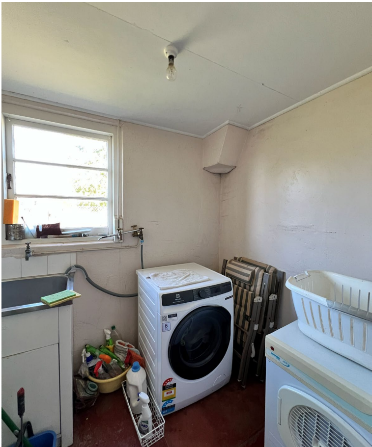
Figure 58 There is a joint separation between plasterboard.
