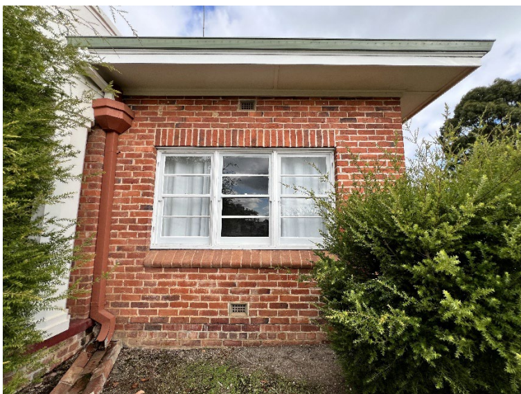
Figure 23 3 combined double hung sash windows. Casement flyscreen missing.
