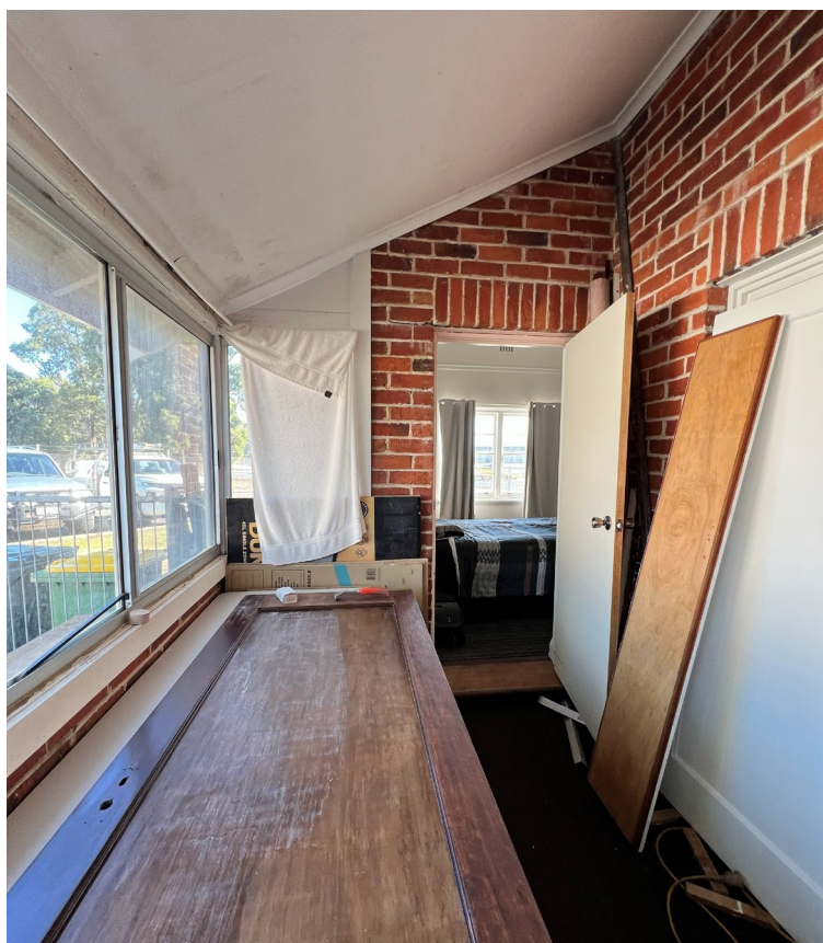
Figure 53 View of sleepout with the bedroom on the background. Small section of asbestos cement sheeting above window.
