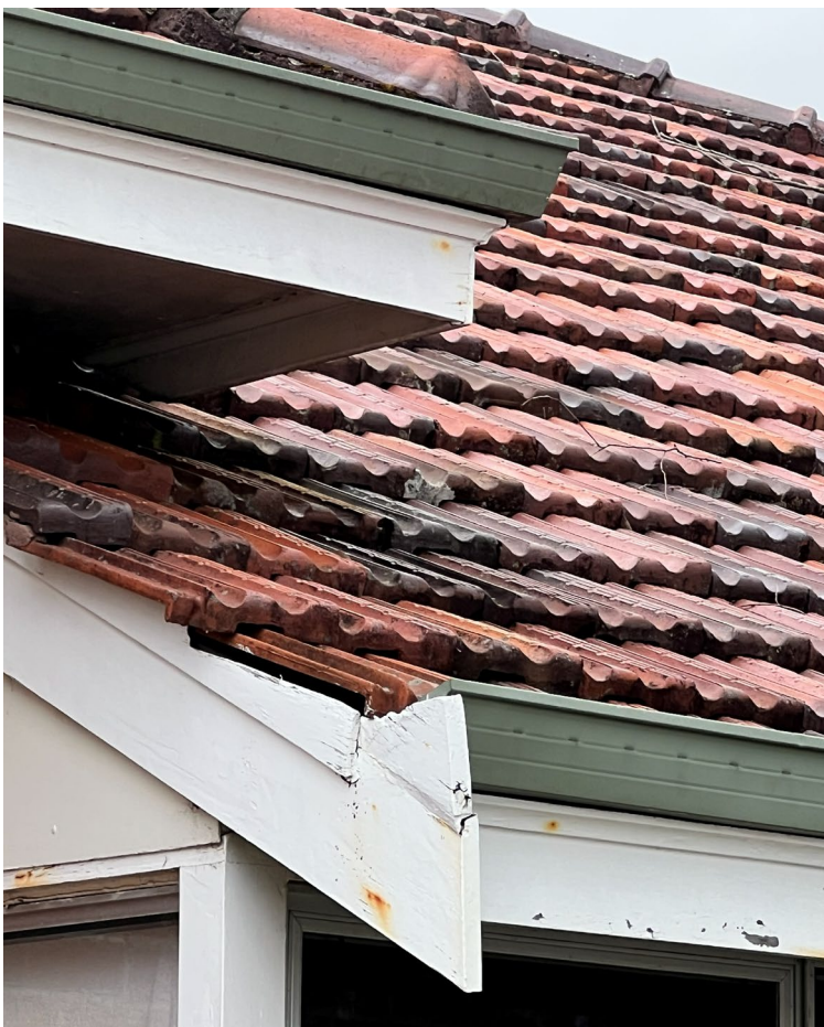
Figure 12 The end roof tile is broken causing water ingress. Timber rot is present at the ends of timber bargeboard. Timber fixings are corroded.
