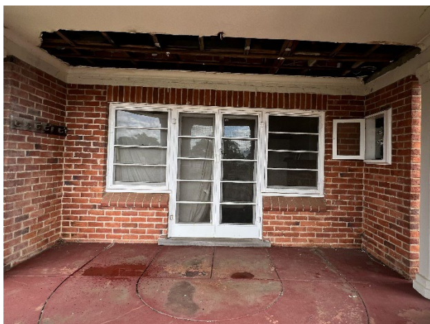
Figure 23 View of glazed door and windows on the eastern façade, and damage to the portico ceiling.
