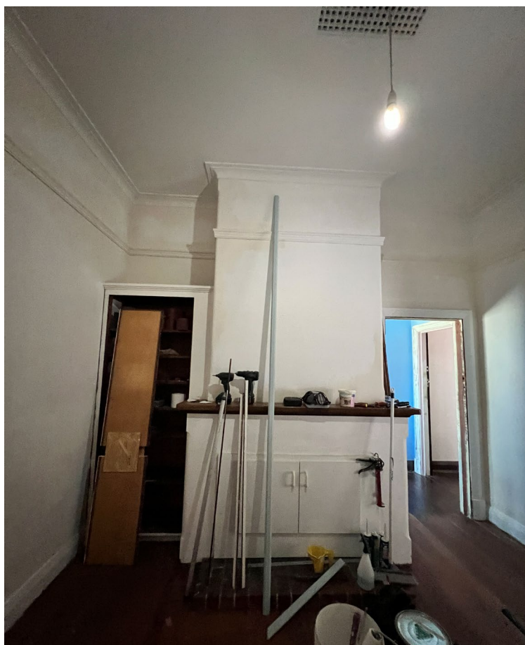
Figure 35 View of consulting room. Firebox fitted with cabinetry.
