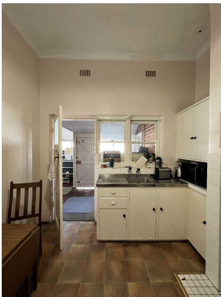
Figure 40 View of kitchen. There is significant water damage to ceiling. Kitchen cabinetry is intact.
