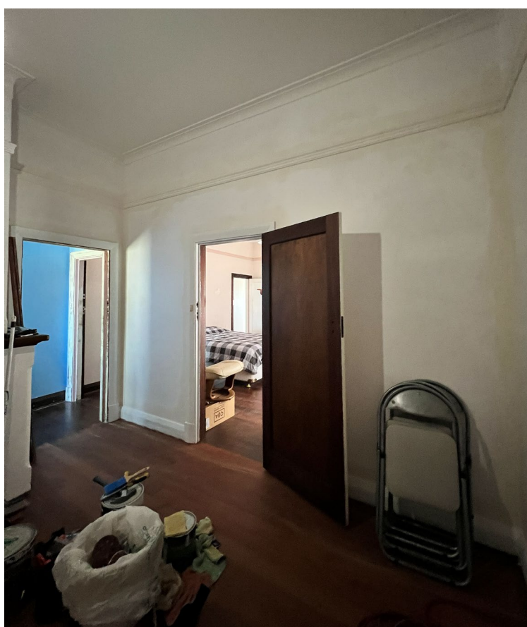
Figure 36 Timber floorboards have been lightly sanded. Scuff marks and stains on walls.
