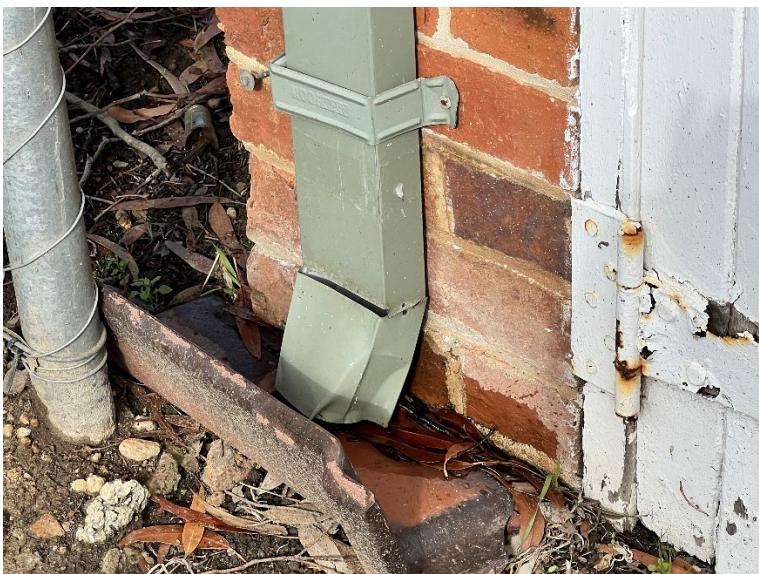
Figure 17 Damaged downpipe discharging onto roof tile. Hinge to garage door is heavily corroded.
