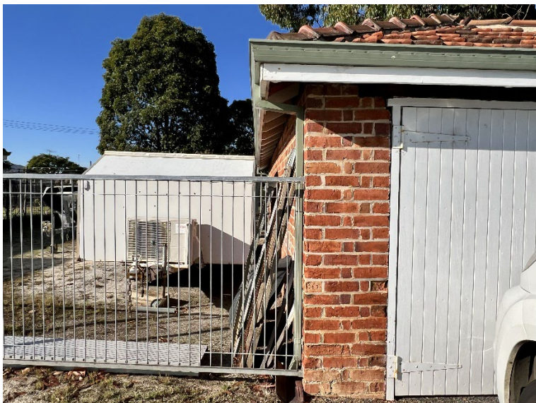
Figure 7 Partial view of the west elevation of garage showing fretting of bricks.
