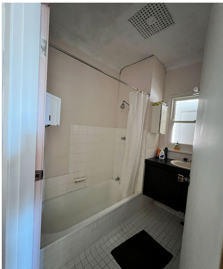
Figure 45 Plaster ceiling to bath is heavily stained. Floor and wall tiles are intact.
