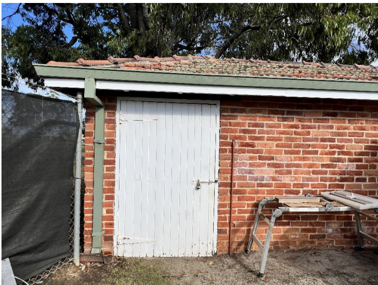
Figure 6 Partial view of north elevation of garage. Lichen growth can be seen on roof tiles.
