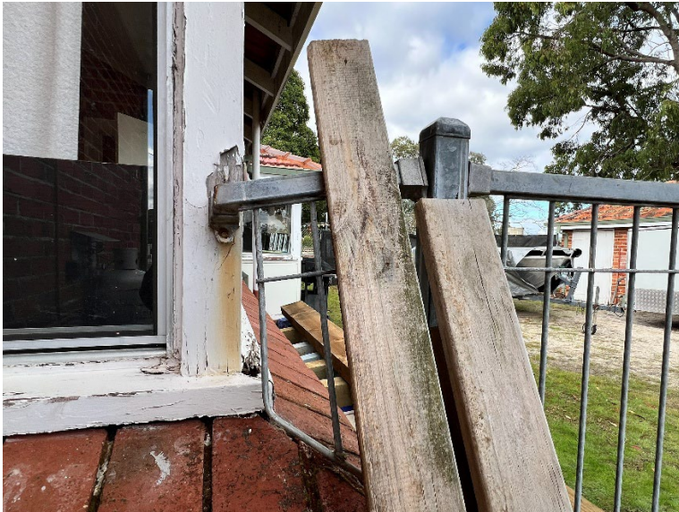
Figure 16 Badly deteriorated timber post attributed to weathering and corroded fence fixing. Mortar missing on brick sill.
