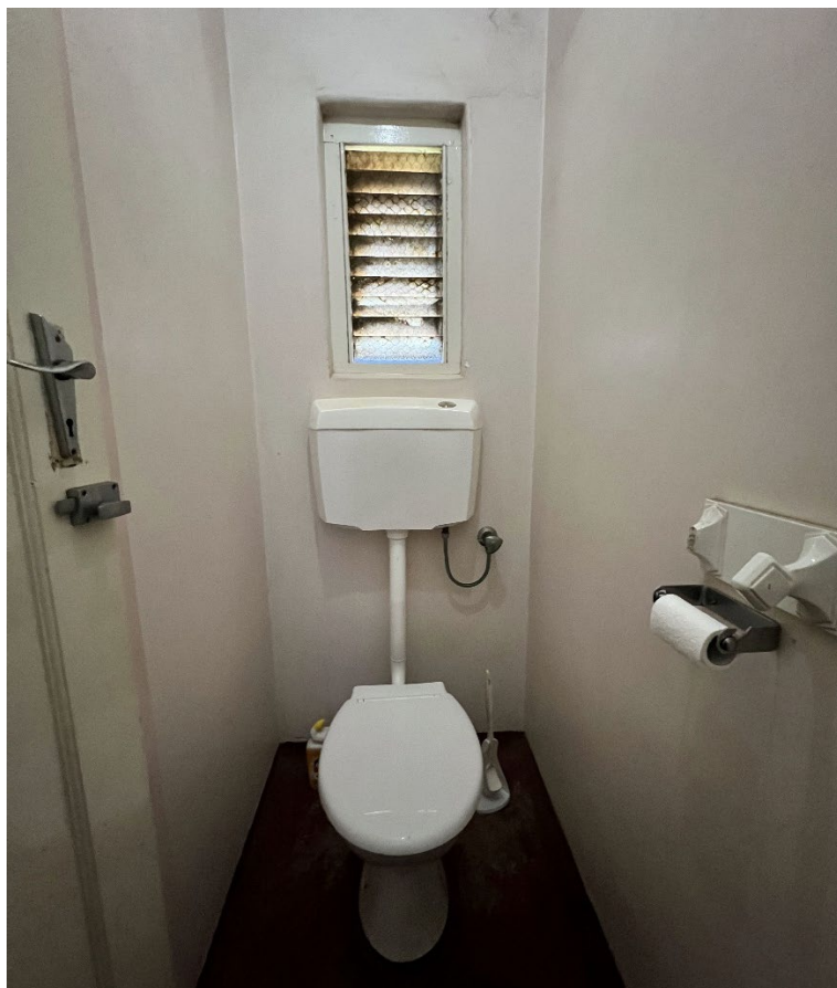
Figure 51 Accumulation of dirt and grime on glass louvres. Original toilet roll holder is broken.
