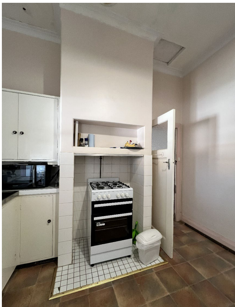
Figure 41 Tiled fireplace. There is a broken tile at the corner of hearth.
