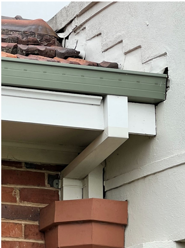
Figure 9 Holes on render and step flashings. Missing timber scotia.
