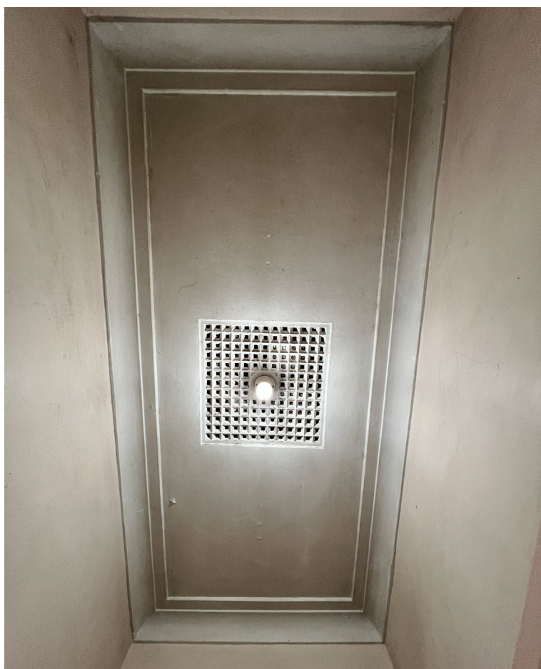
Figure 52 Plaster ceiling to WC1 is heavily soiled.
