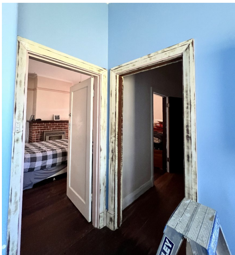
Figure 39 Door architraves to be repainted.
