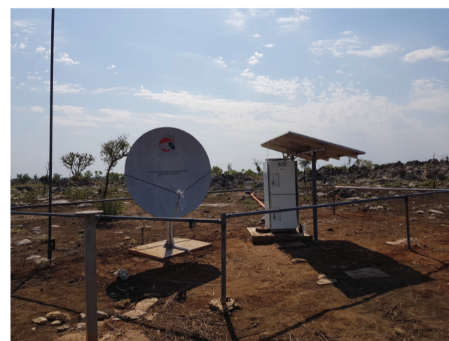
Image courtesy of Geoscience Australia. Image outlines an indicative setup of a seismic monitoring station.
