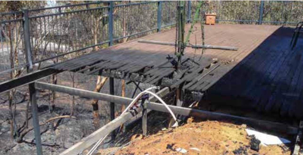
Below: Deck damage as a consequence of being constructed from inappropriate materials for the potential BAL.
