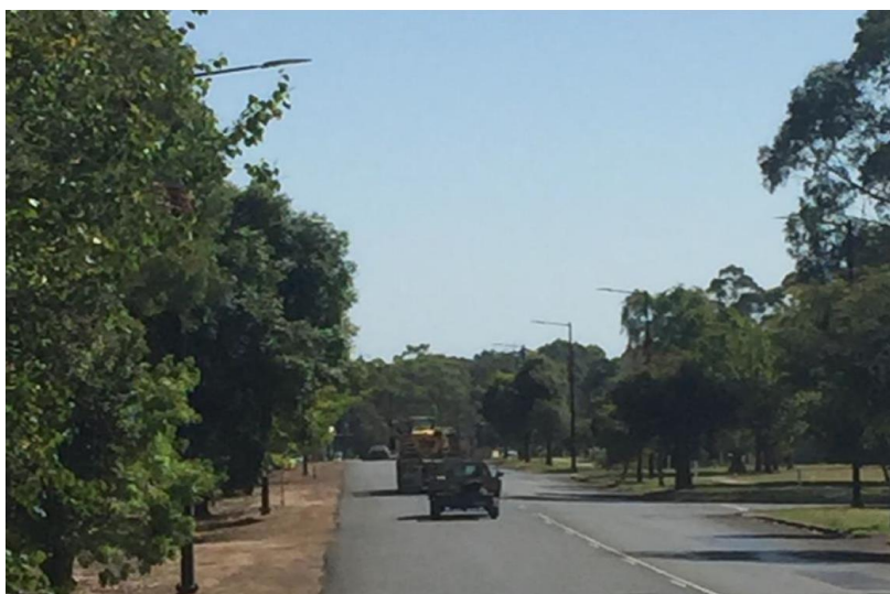
Figure 2.1 Removal of Overhead Power Lines and New Street Lighting along Mottram Street
